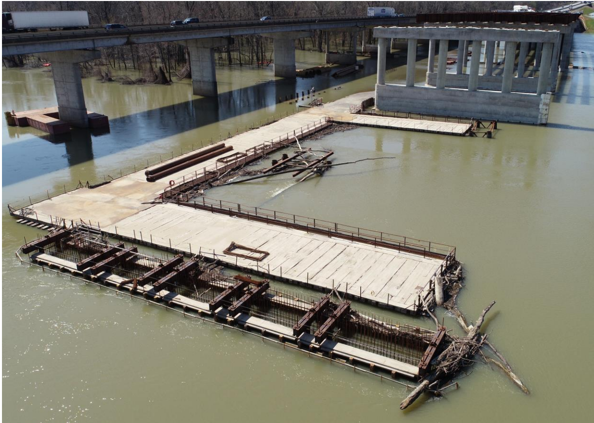
2. Example of 2019 flood conditions near normal river channel, photo taken 3-18-2019, 25 days after cresting 2' over this trestle
