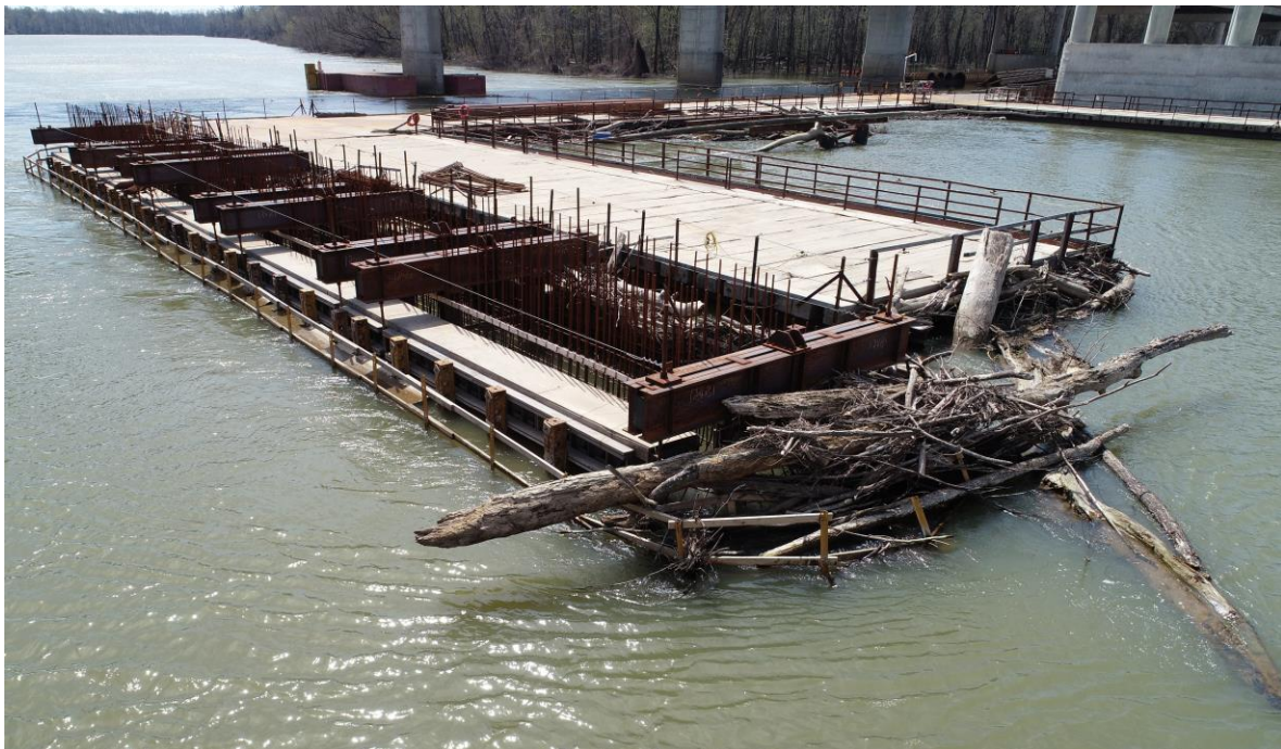
3. Close up of built up debris from 2019 flood conditions, photo taken 3-28-2019
