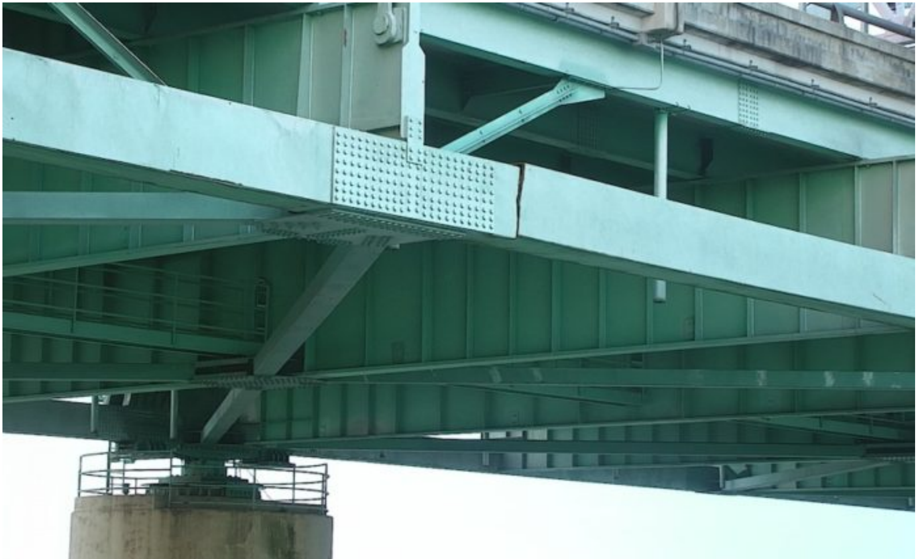
Recent 2021 Photo of Fracture
